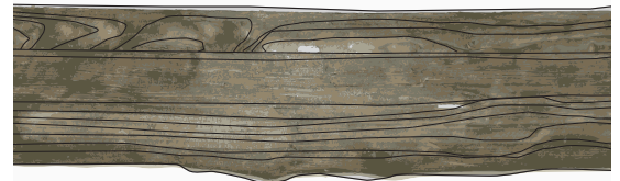
Figure 16.2 Glulam beam without significant singularities after a fire
