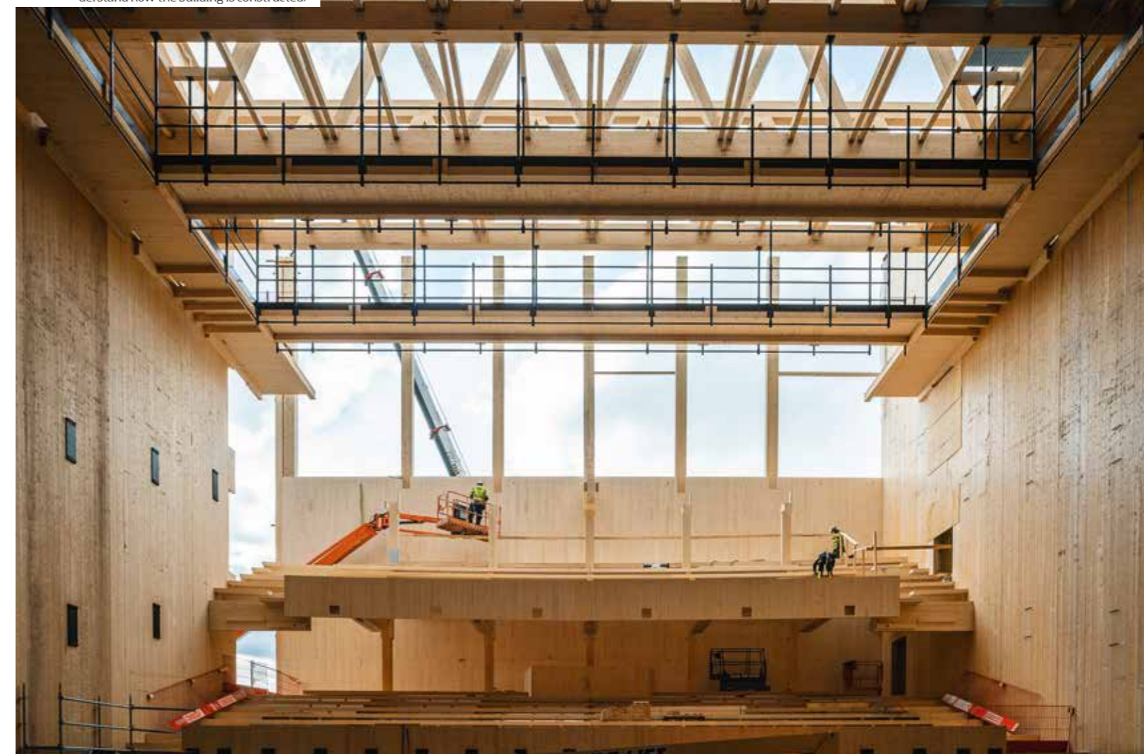
Locally based prefabrication ensured short processes during construction. The architects wanted to make it easy to understand how the building is constructed.
