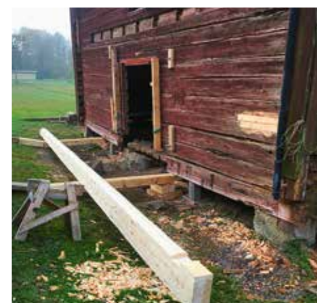
Parts can be replaced in log-built structures which can also be dismantled and erected elsewhere. Pictured is a log-built storehouse that is having its sill log replaced.
