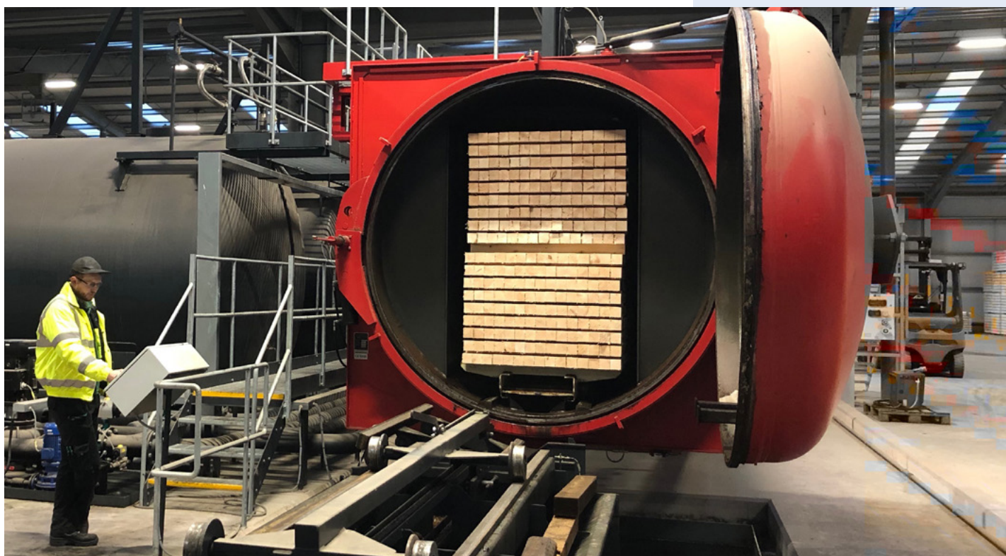
A typical wood preservative pressure treatment plant. Photo courtesy of James Jones & Sons Ltd.
